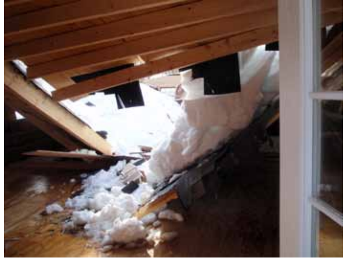
inside the collapsed building
