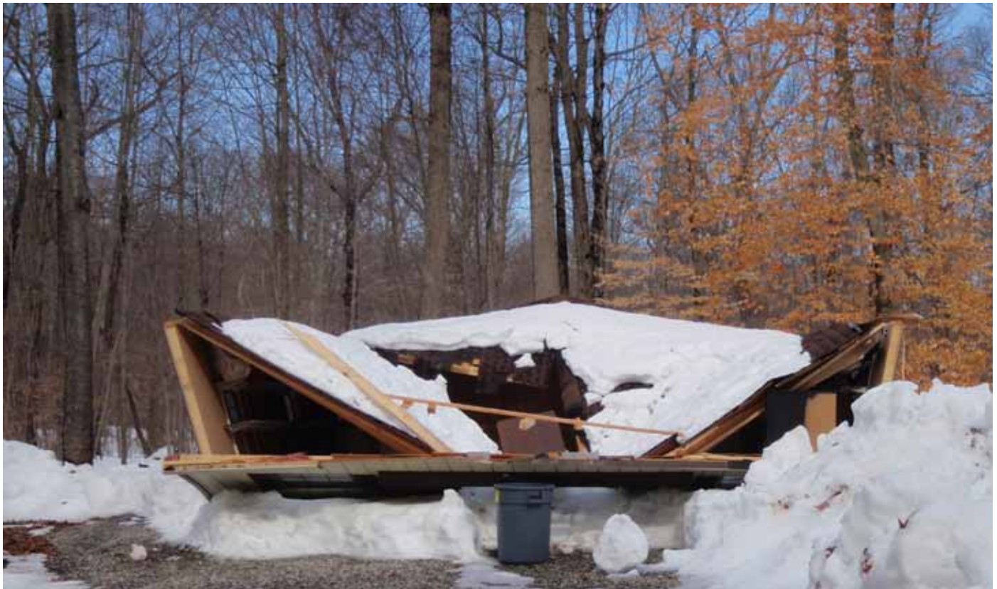
collapsed building from the front
